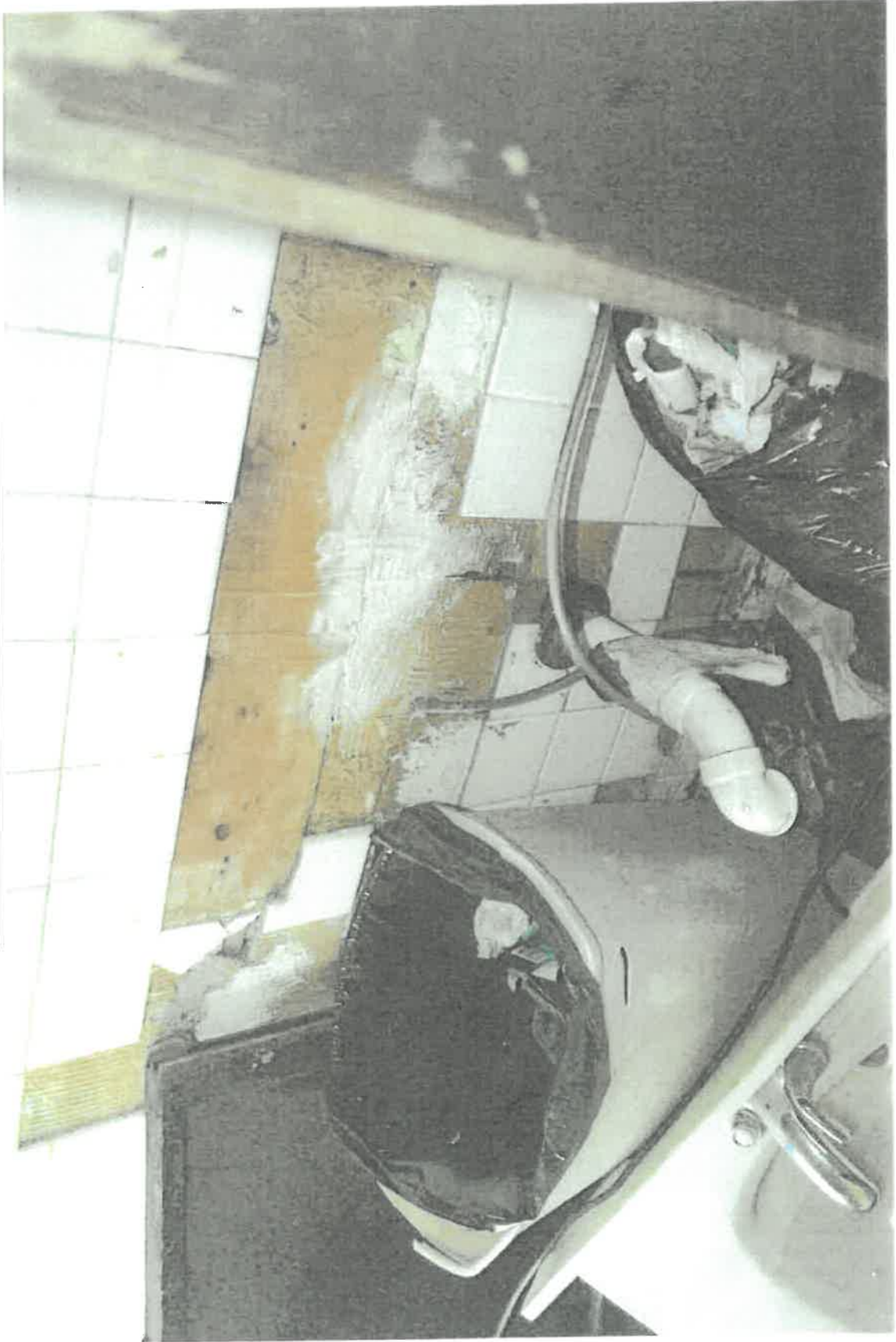
2 ND DIVISION BATHROOM – SINK IS REMOVED FROM THE WALL.
