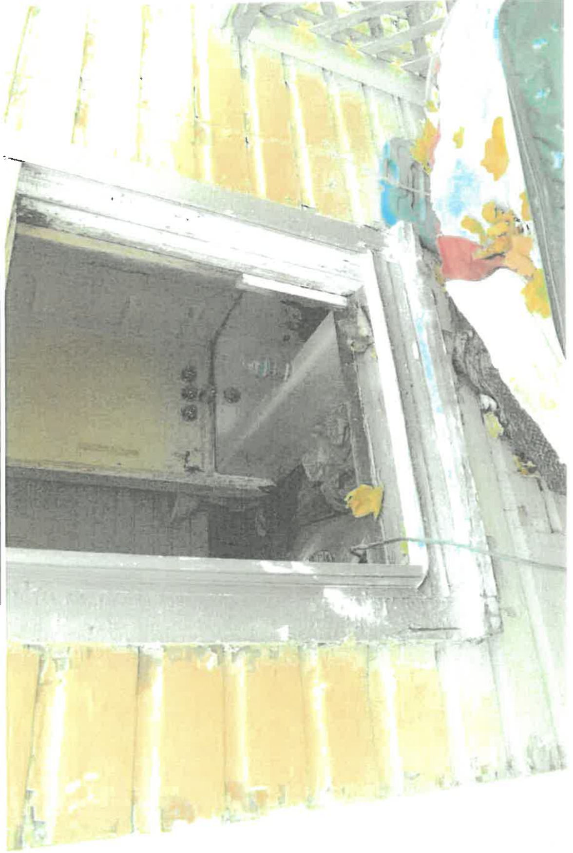
2 ND DIVISION BATHROOM. PHOTO TAKEN FROM OUTSIDE. WINDOW IS BROKEN.
